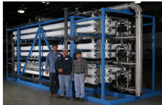
1,050 GPM Reverse Osmosis Unit
