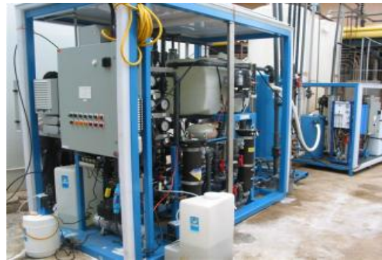
Figure 1: Ultrafiltration Pilot Unit
