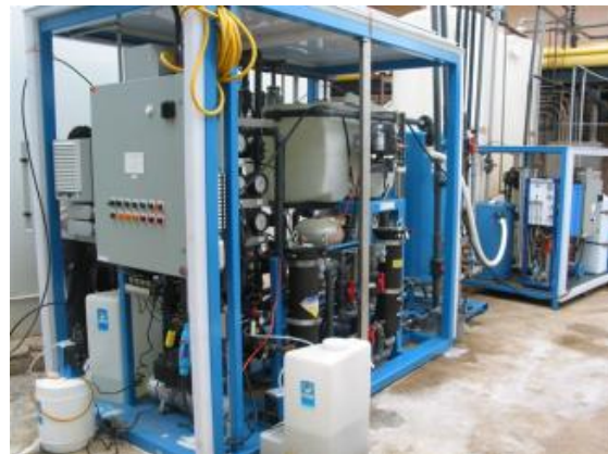
Figure 4: Pilot Rig for Silt Density Index, Ion Exchange, and UF Testing
