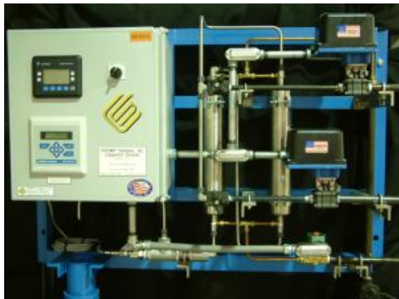
Crown Two-Station Blowdown Controller with Sample Coolers
