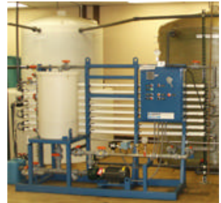
CROWN's objective was the successful implementation of a tubular wastewater ultrafiltration system, reducing the amount of waste hauled off-site by up to 95%.
