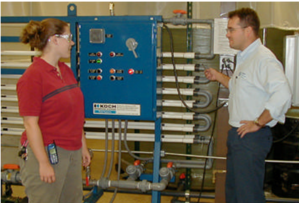
Jenny Leverett, left, is CROWN's full time environmental specialist at the Dayton facility. Leverett is responsible for conditioning the wastewater to make it acceptable for disposal to the local municipal wastewater treatment plant. At right is Randy Hill, service manager for CROWN Solutions, Inc.
